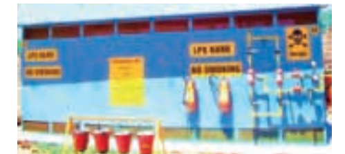
Like everything else at our projects, the Gas Bank at Amarbagh is an example of safety, meticulousness and aesthetics
